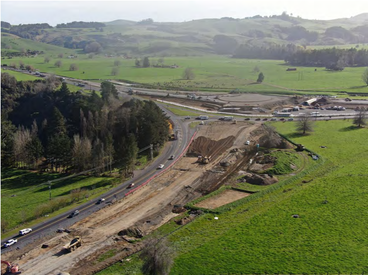
Southern approach to SH1/SH29 for the new roundabout. Image courtesy of NZTA
