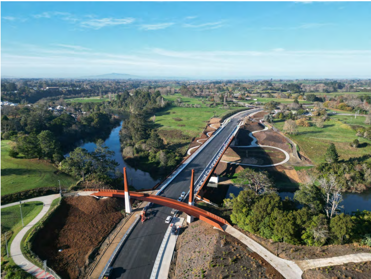
Construction of a new bridge over the Waikato River and surrounding transport network is under way in the Peacocke neighbourhood, Hamilton. Photo courtesy of BBO.
