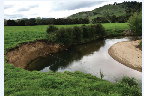
Rocks were placed along this outer corner of Wharekawa River to help prevent erosion.
