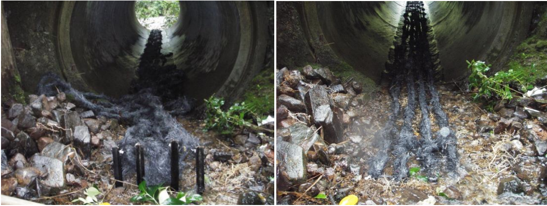
Upstream end. Install with metal stakes and thread rope through galvanised 'D' shackles that fit through top hole (left photo). Once threaded through hammer into bed and cover over (right photo)
