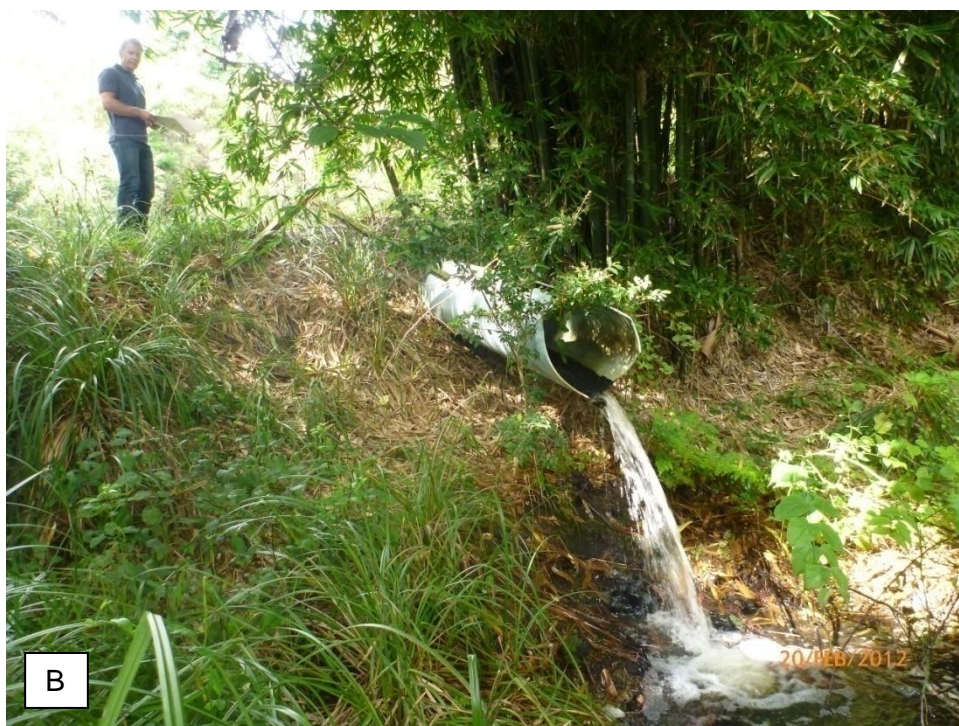
Figure 1: A,B. Poorly installed culverts on a tributary of the Mangakotukutuku stream in urban Hamilton. In the lower example a perch height in excess of 1m combined with a 12m pipe length and pipe gradient in excess of 10 makes this a formidable barrier to even the most aggressive upstream climbing species.
