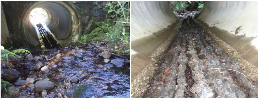
Completed retrofit looking downstream (left photo) and upstream from within culvert (right photo). Note 'swimming lanes' formed by ropes.
